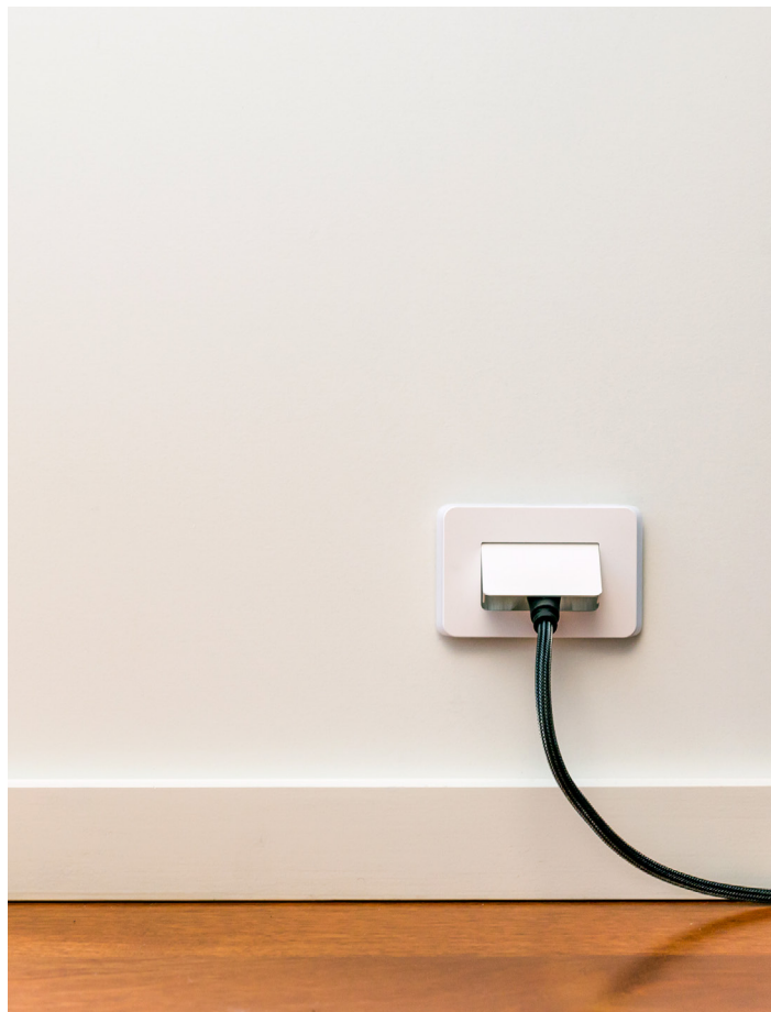
Aesthetically appealing cable management
