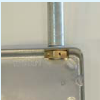
Connection to steel conduit
