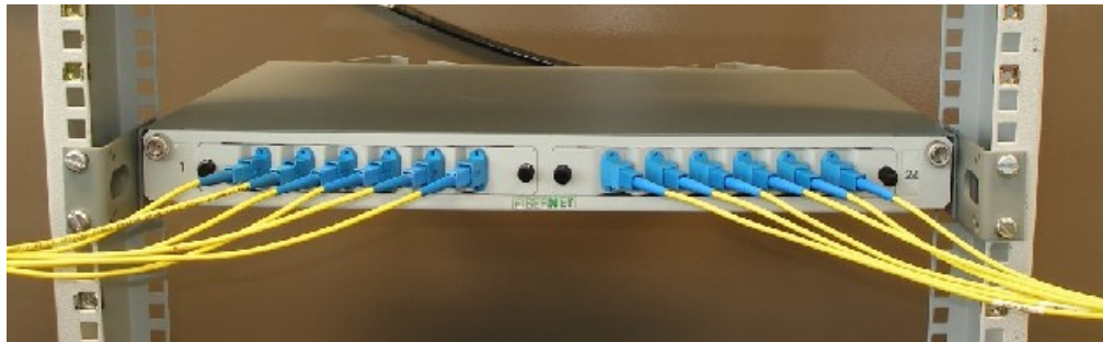
Figure 17. Patchcord routing from the front of cabinet
