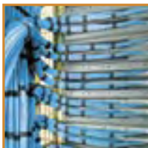
Data Cabinet Installations
