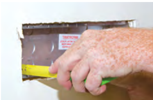
Step 4. Ensuring wall box is a minimum of 16mm below finished wall surface, screw-fix to wall studs.
