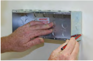
Step 1. Mark out location of multi-gang wall box (use outside of wall box as a guide).
